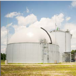
Biogas Plant Berkeley County USA
